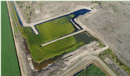
The end wetland result. The system was designed with earthen berms to direct water flow, a sediment pit at the larger inlet, and a leaky rockwall at the outlet.
